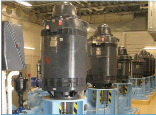
The motors atop these vertical hollow-shaft pumps (at the Reverse Osmosis Water Treatment Center in Hutchinson, Kansas) provide thrust to the pumps' drive ends.
